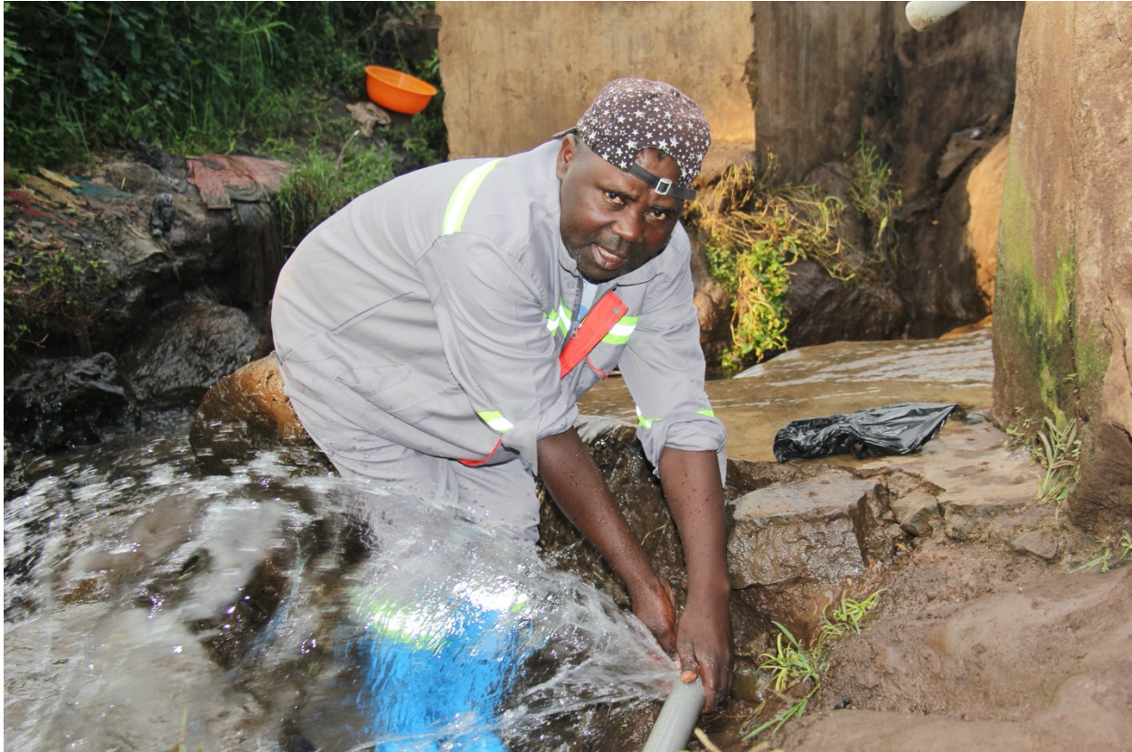
Maintenance of the NYABIREHE drinking water pipe by ASUREP KATANA's senior technician, Mr. Douglas KAHUGUBA. Photo credit: Mercy Corps/Elie Mukengere
