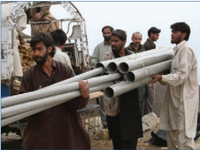
Residents of northern Pakistan's Konch Valley unload supplies provided by USAID for building sanitation facilities near their homes.
