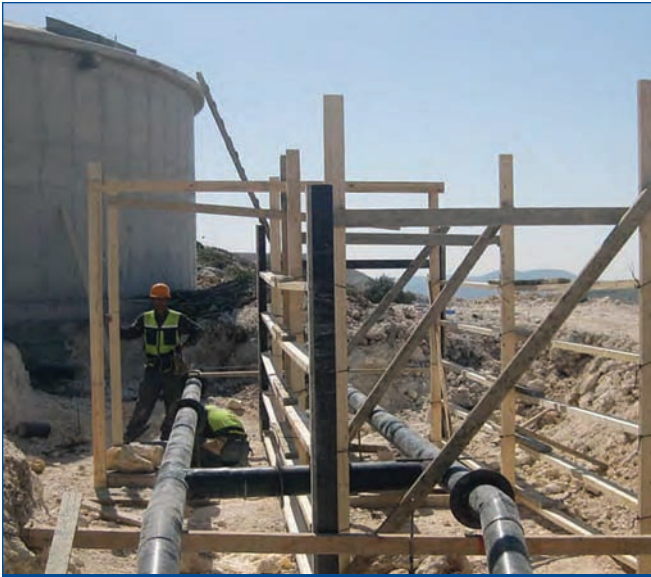
Reservoir construction is a major activity of USAID's Water Resources and Infrastructure Program in the West Bank and Gaza.
