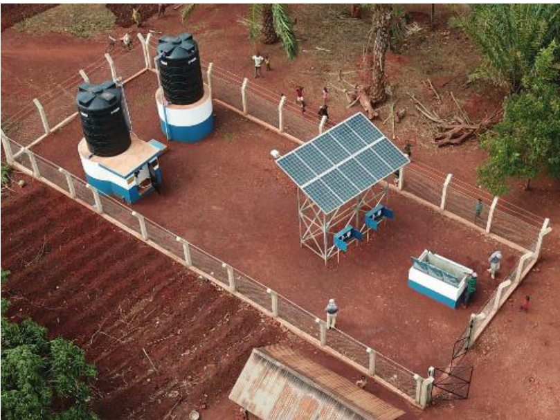
Figure 5. Community-scale solar-powered water pumping system in Tanzania (Source:Water Mission)
