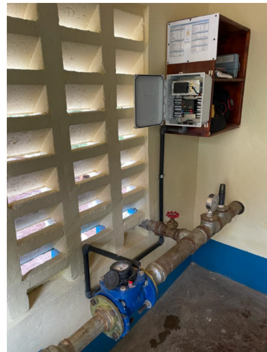
Figure 19. Water Mission SatWater Communicator connected to a pulse water meter in a pumphouse (Source: Water Mission)
