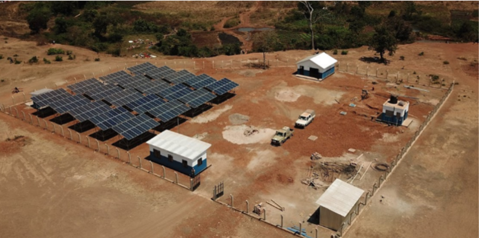
Figure 6. Solar pumping system installed in a refugee camp in Tanzania (Source:Water Mission)
